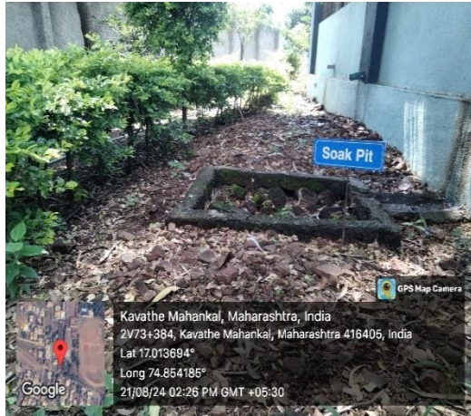
Soak pit for every laboratory drainage
